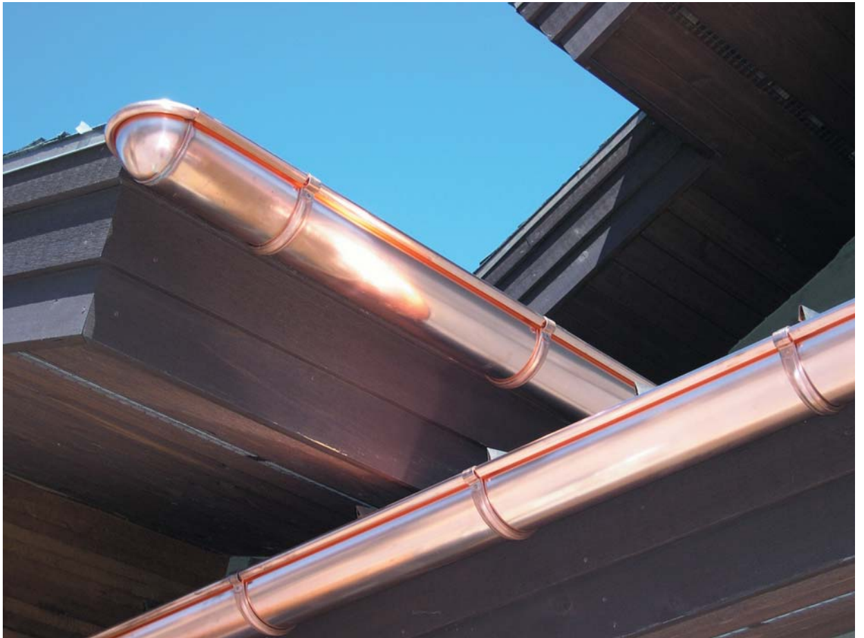
Park City Rain Gutter is the U.S. distributor for the Italian-made Minoletti copper gutter system. This typical installation shows a 6-in. single-bead half-round gutter with a round end cap. This newly installed gutter will patina beautifully over time, says owner Gene Stucky.
