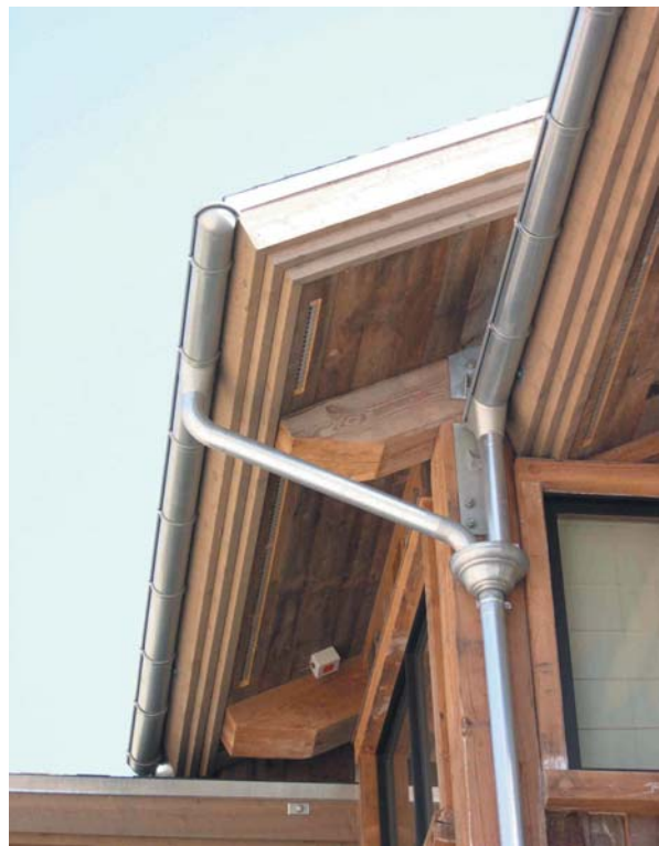
This zinc gutter system supplied by Park City Rain Gutter was designed to match the galvanized trim and structural connecting plates on a mountain home.
